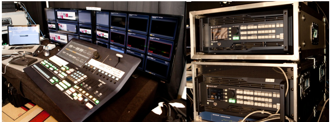
Vertige™ controller and the two Ascender 48s linked in the control room
