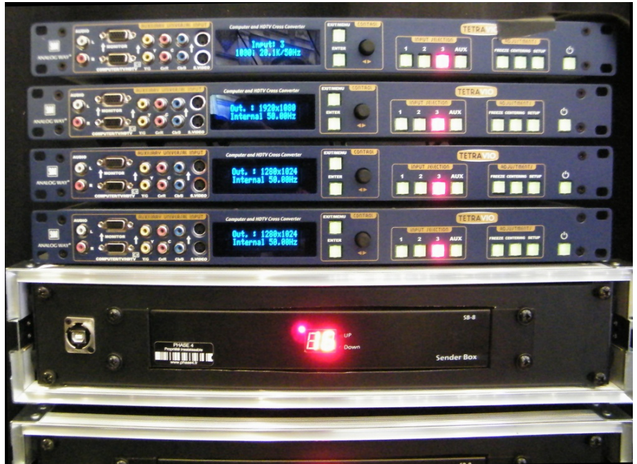
4 Tetra-VIOs in the control room of La Plaine St Denis studios - Paris
